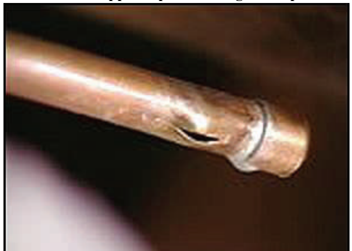
Frozen Copper Pipes will bulge and split
